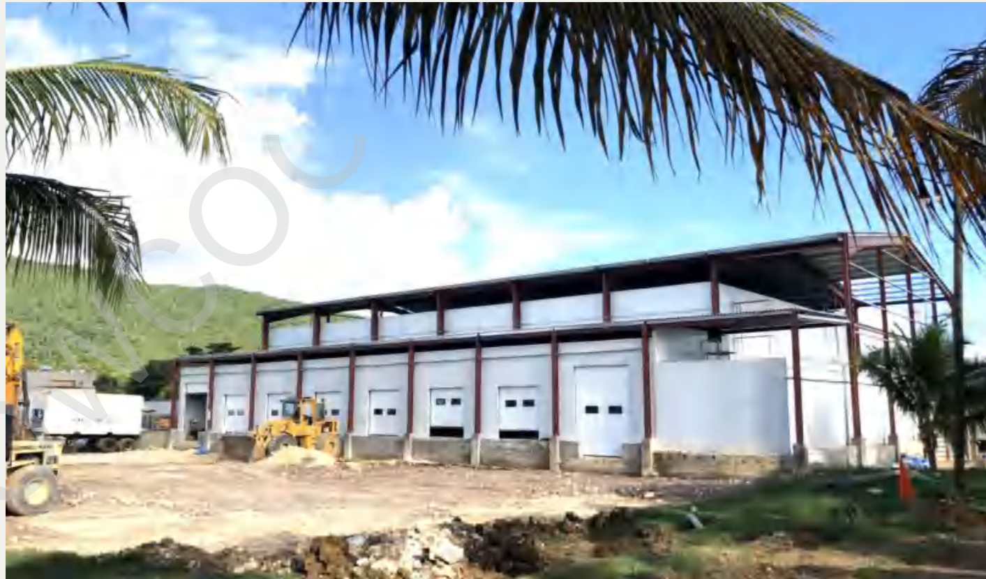
Jamaica 3000 ton cold storage project
